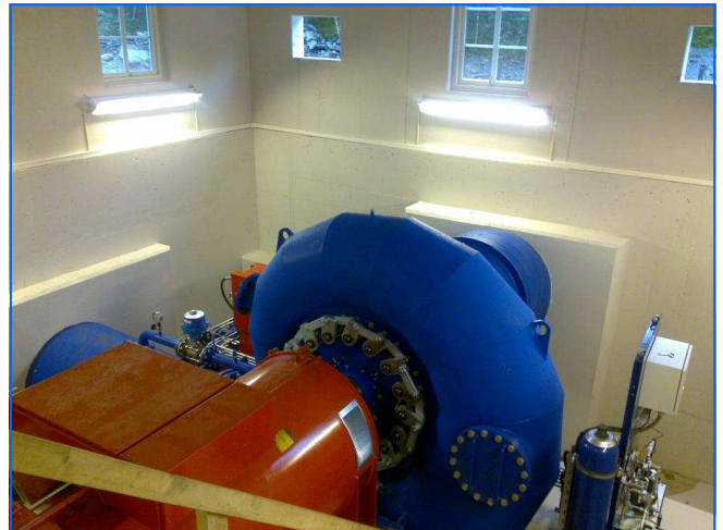
Krafthaus Power house
