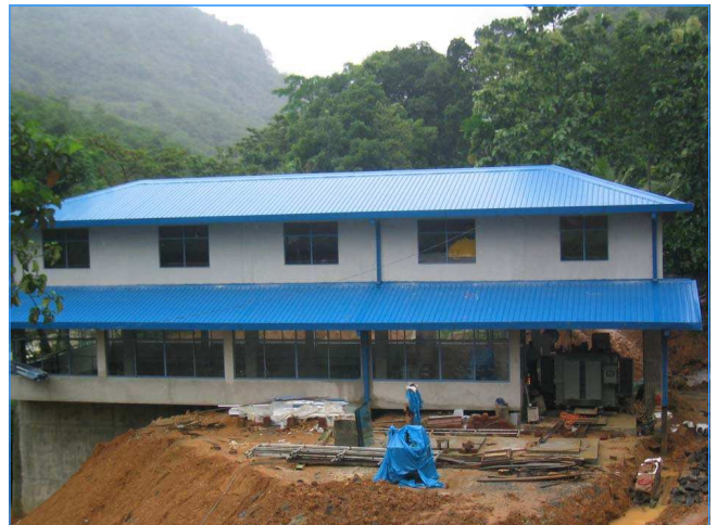
Baustelle in Sri Lanka, Turbinenhaus Construction site in Sri Lanka, turbine house
