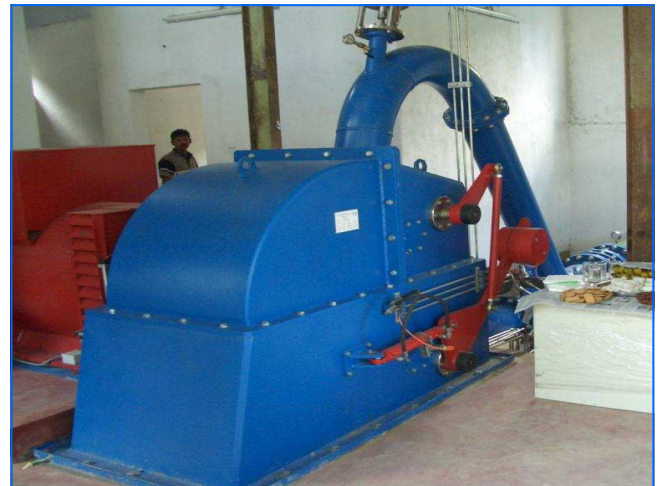
Installierte Pelton Turbine installed Pelton Turbine
